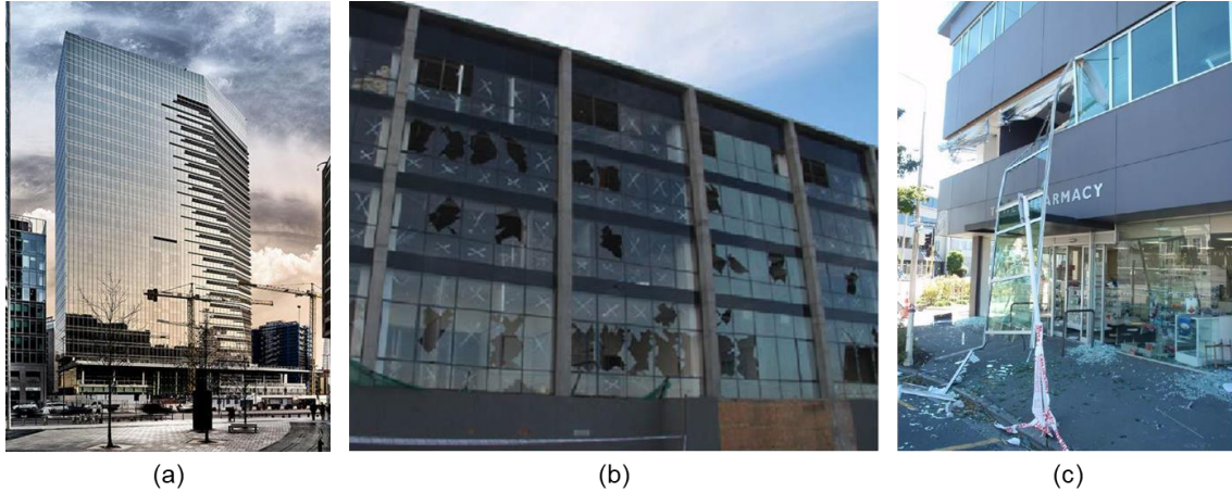
Figure 1. (a) Example of unitised glass curtain walls installed in a high-rise building – GIOIA 22 tower in Milan, Italy (by Permasteelisa Group); Seismic damage to glazed façades: (b) 2010 Chile earthquake (FEMA E-74), (c) 2011 Christchurch earthquake (Baird et al. , 2011).
